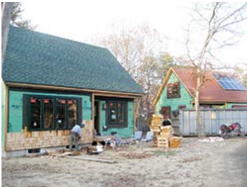
Workers finish up a house at Jenney Way. Photos Courtesy IAHF. Click photo for larger version.
